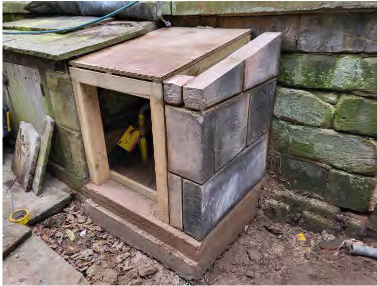
Figure 1: Gas Meter Enclosure - Masonry Constructed.
